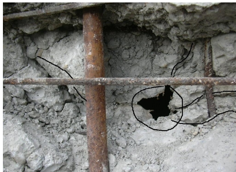
Fig. 4. Local cavities and in-deep reinforcement corrosion
