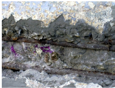
Fig. 6. In-deep reinforcement corrosion
