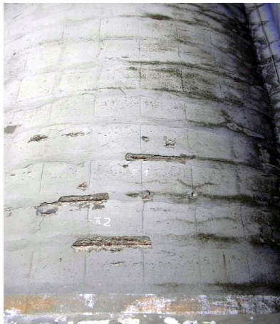
Fig. 5. Deteriorations on external cell surface
