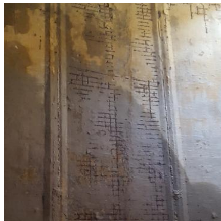
Fig. 11. Degraded reinforced concrete wall
