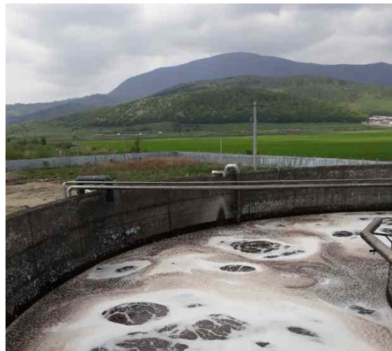
Fig. 7. The wastewater decanter in-service
