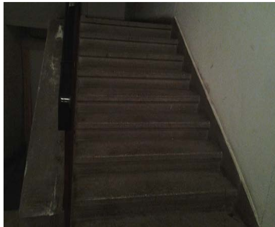
Fig. 7. 'When the lift is out of order, going up the stairs to the third floor is tormenting' (Reproduced with the permission of Hospice Casa Speranței Braşov)
